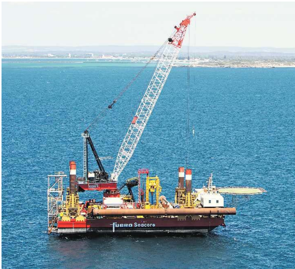
Making waves: The vessel will put in place the foundations for Carnegie's ambitious energy project off Garden Island
