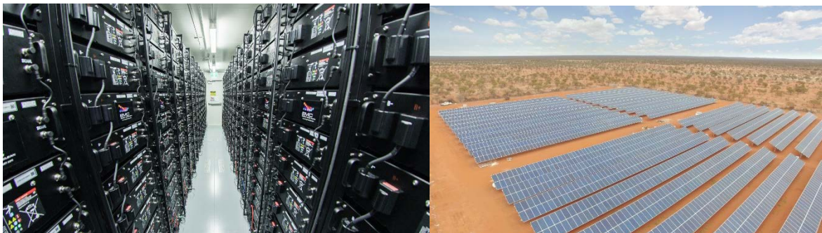
EMC’s utility battery system for Synergy’s Alkimos project (left) and solar array for CSIRO’s Square Kilometre Array (right)
