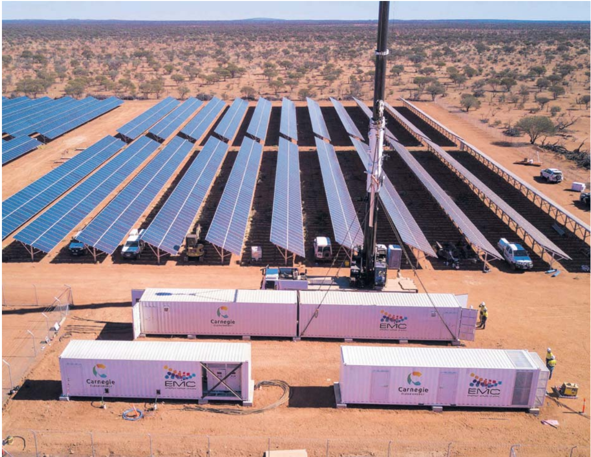
Batteries built by Carnegie Clean Energy are hooked up to solar cells at the Square Kilometre Array.
